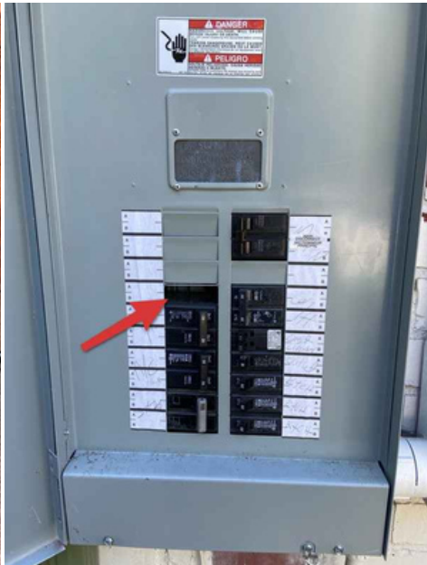
Missing Knockout Plug
